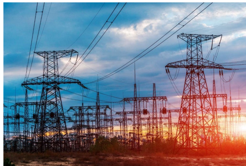
Power line fault
